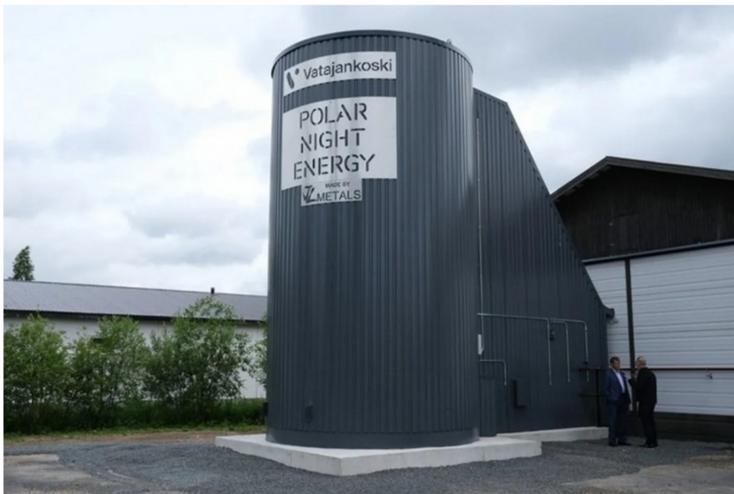
The sand battery. Image credit: Polar Night Energy
